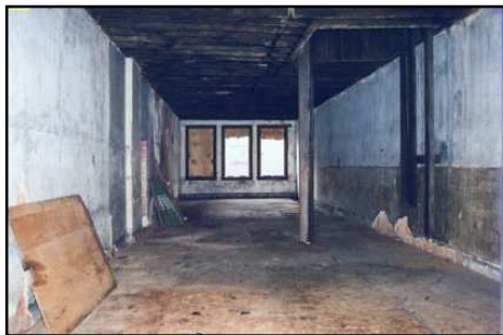
Figure 26 – "Kinsey Flats" When the developer purchased the "Kinsey Flats" buildings in 2002, the buildings were in serious disrepair and had to be stabilized before rehabilitation could begin. Source: ULI: Development Case Studies
